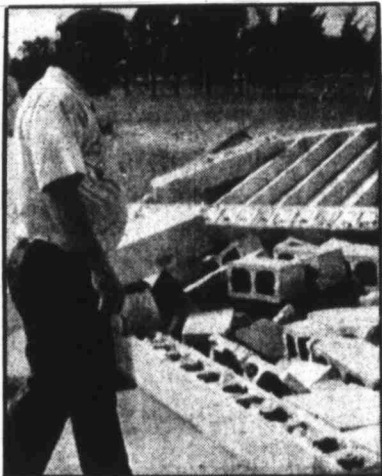
STORM DAMAGED DUGOUT
