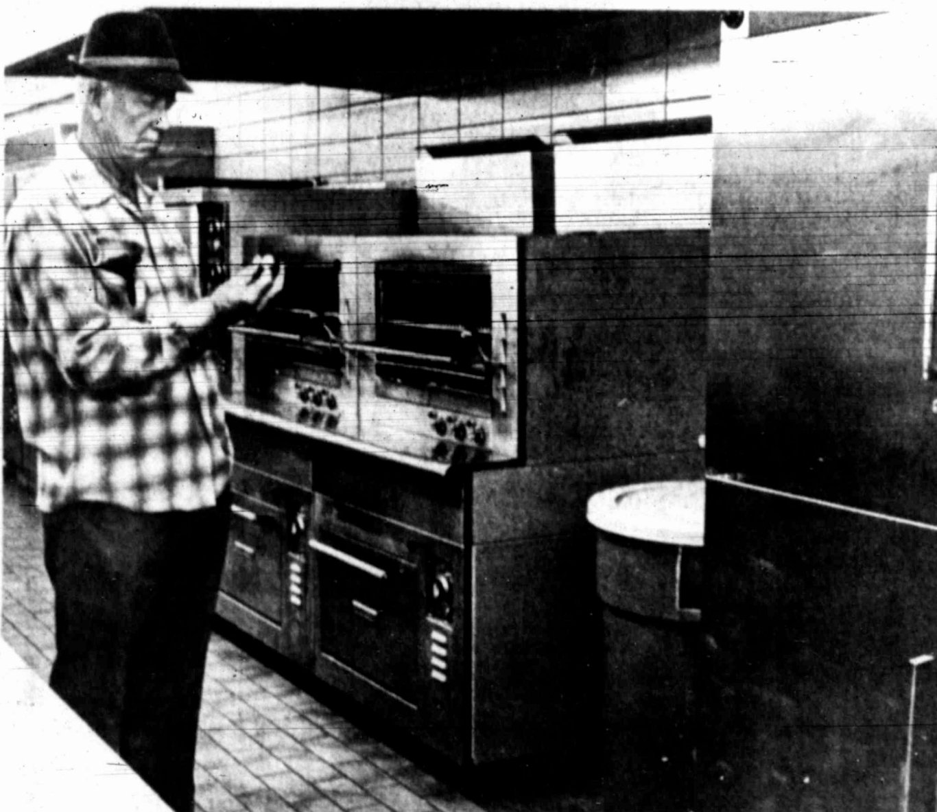
Efficient warming facilities in Harvey Hall's kitchen will accommodate a banquet capacity of
