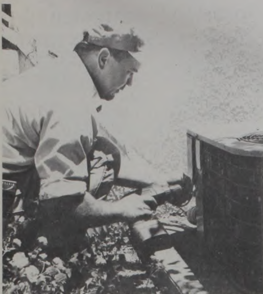
EXTREMELY HOT WEATHER with temperature highs peaking in the 100s is hard on people and animals, as well as air conditioners. Curtis Hesse of Hesse Heat and Air services one of many units that succumbed to high temperatures and overwork. Hesse recommends that homeowners practice preventive measures by changing or checking air filters monthly; oiling motors inside and out; and having it checked regularly by a service technician.
