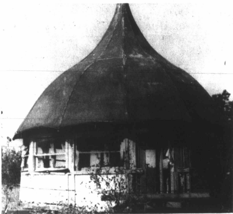
A DETERIORATING ROUNDTOP, with most of the back side of the structure missing, sits behind the city barn. Kiwanians hope to interest local residents in a Save The Roundtop effort.
