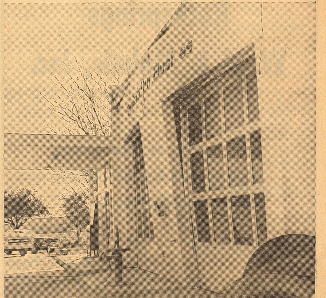
AN EARLY MORNING EXPLOSION pushed the front walls of W. H. Hill's service station several inches out near the top of the building. The explosion apparently occurred when fumes
