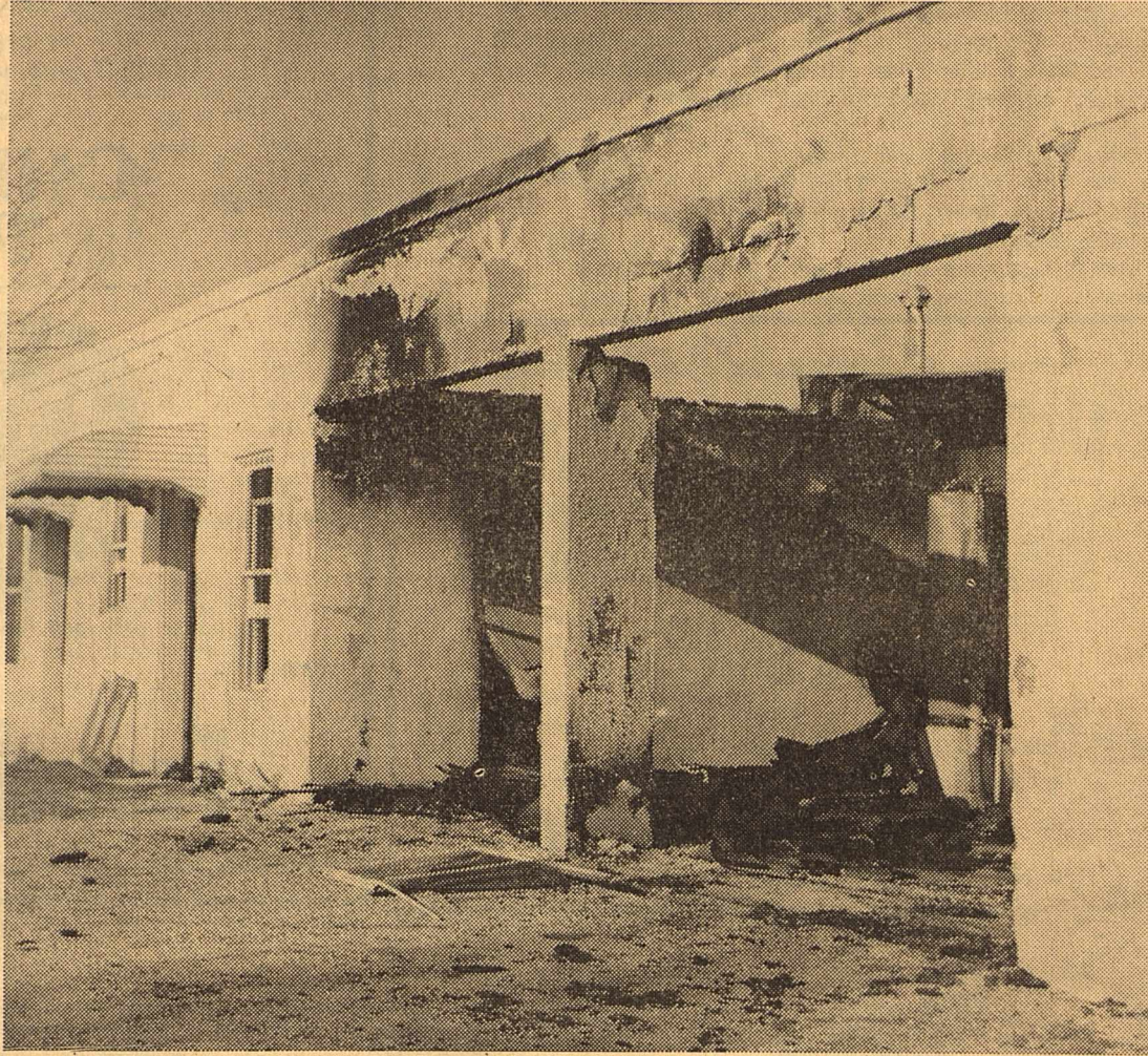
THIS CARPORT AT ZOLA'S COURTS was the center of the devastating fire last week. The flames are believed to have broken out in
