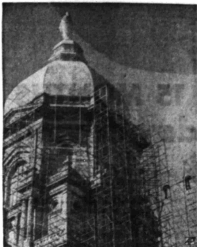
NEW COVER —Scaffolding is set around the Golden Dome at the University of Notre Dame prior to replacing the dome's sheet metal base and covering it with gold leaf.
