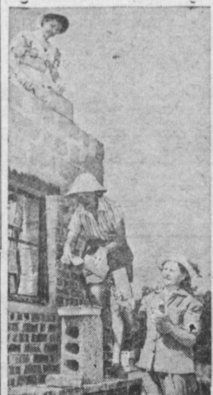
THIS IS THE HOUSE! . . . Out at Lemont, Ill., a house is rising which is different than the house that Jack built in the nursery rhyme, because much of the work is being done by a couple of Janes. Mrs. Joseph Gurski, center, is laying brick on the new family home, assisted by willing friends.
