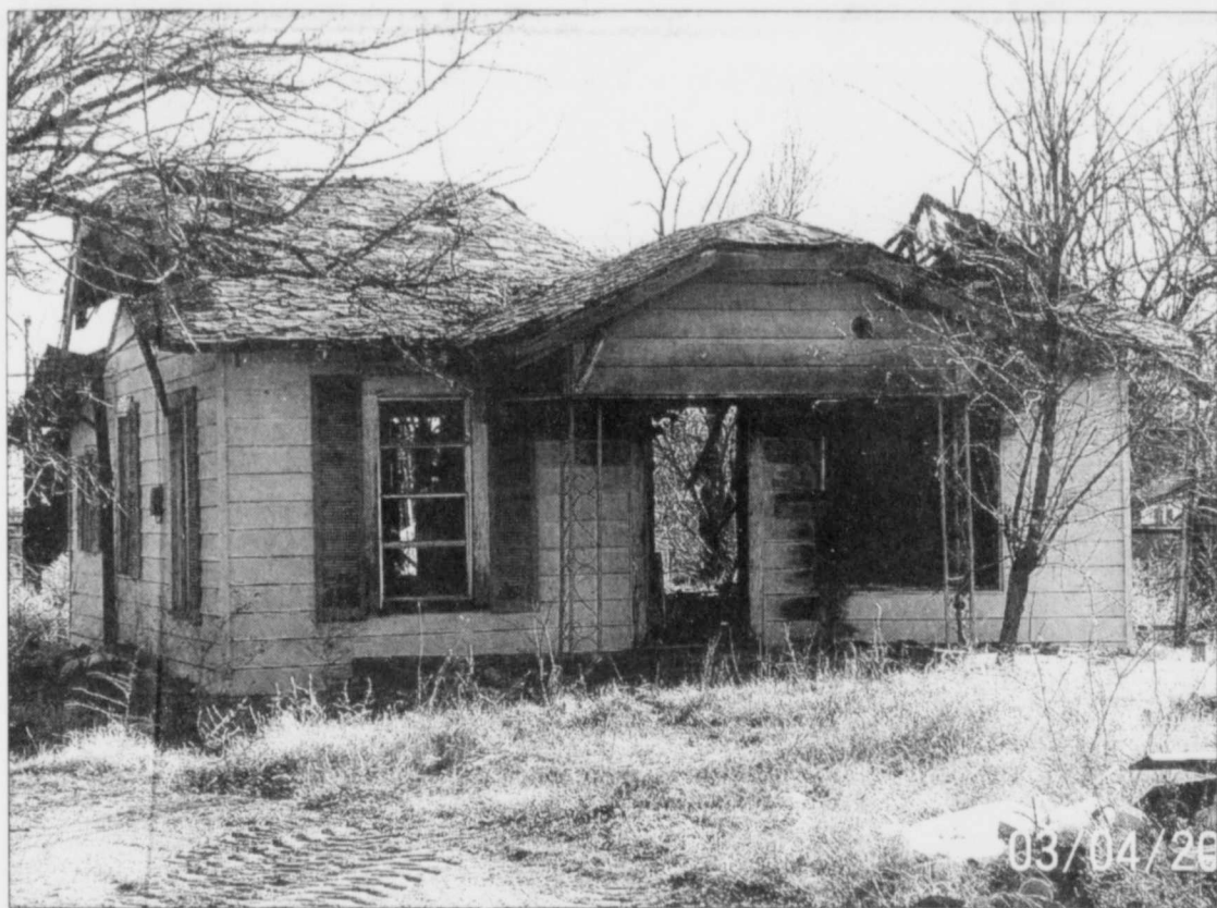
STRUCTURE EYESORES LIKE this one on 7th Street will be the focus of Reclaim Colorado City, a community partnering project to improve the city through code enforcement compliance. Photo courtesy of Colorado City Police Department
