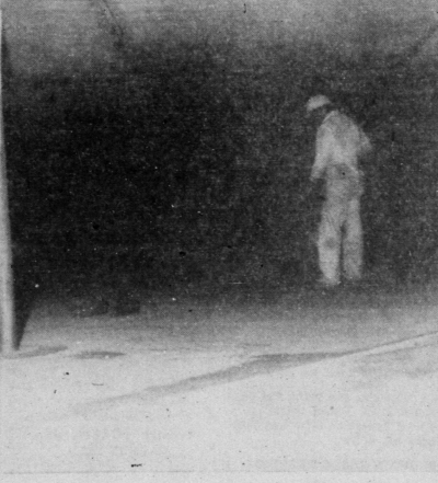
UNDER THE BIG TOP —A workman is sandblasting the bottom of the Mesa tank preparatory to coating it. The tank top under which he works weighs over 100 tons and will float on the oil in the tank. Tank construction started on Jan. 27 and is estimated to cost nearly a quarter of a million dollars. The diameter of the new tank is 134 feet, or more than two average size building lots.
