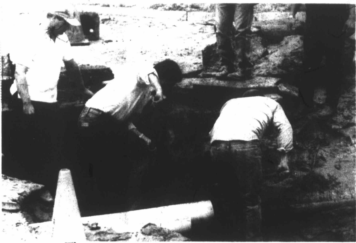
WATER LINE AND PHONE LINE REPAIRS: Workers from the city and Southwestern Bell are shown at the site of a water leak and cable break at the intersection of 4th and Chestnut Wednesday morning. The leak was first discovered at 3:30 a.m. and repairs began at 4 a.m. Phone service was temporarily disrupted in a four-block area that included the City National Bank. Kenneth Rich is operating the backhoe for the city and Jesse Munoz, Jr., is repairing the cable for the phone company.
