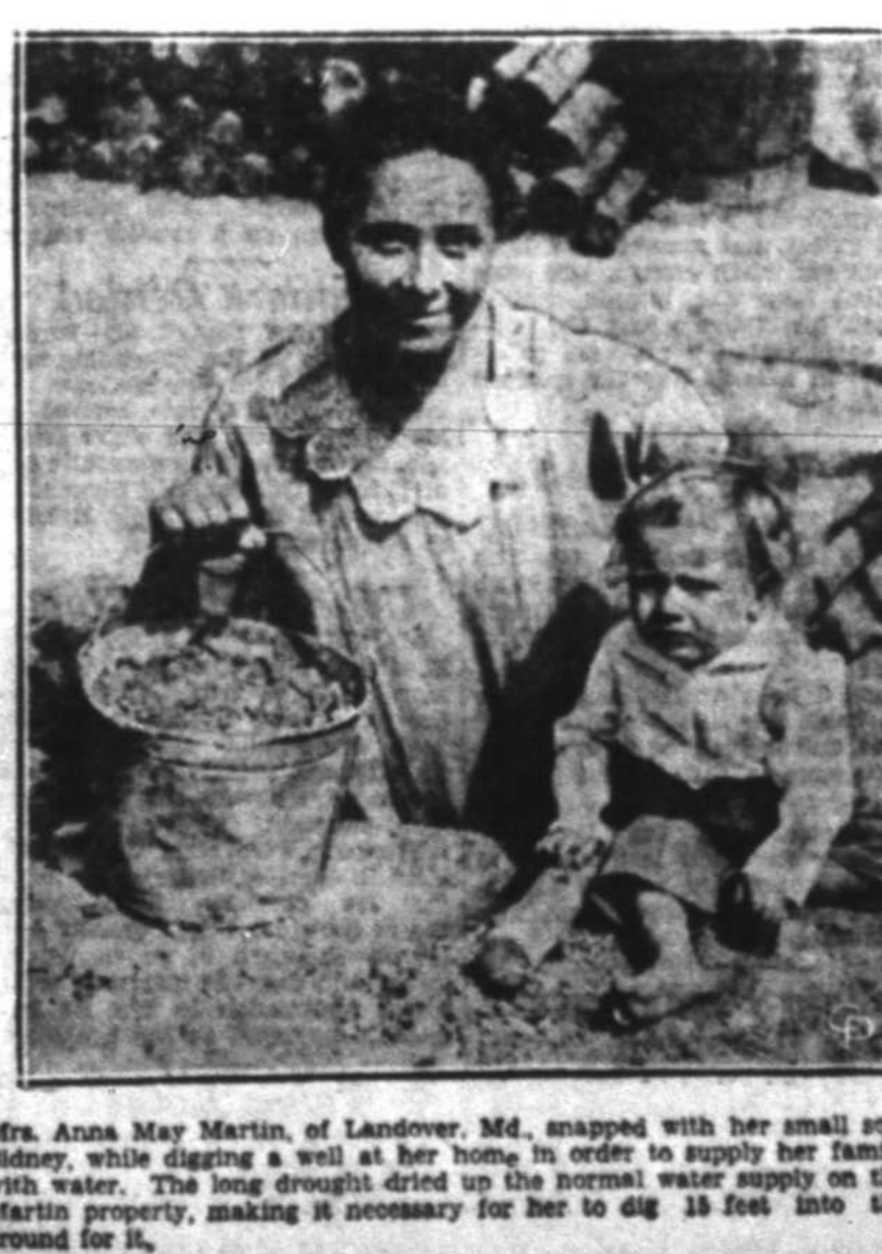
Mrs. Anna May Martin, of Landover, Md., snapped with her small son, Sidney, while digging a well at her home in order to supply her family with water. The long drought dried up the normal water supply on the Martin property, making it necessary for her to dig 15 feet into the ground for it.
