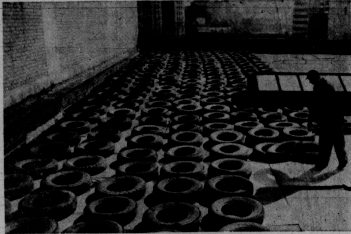
Tiring Work Worker lays down hundreds of rubber tires on a Rochester, N. Y., rooftop. The old tires and plywood sheeting are used as protection against falling debris from the adjacent building being torn down.
