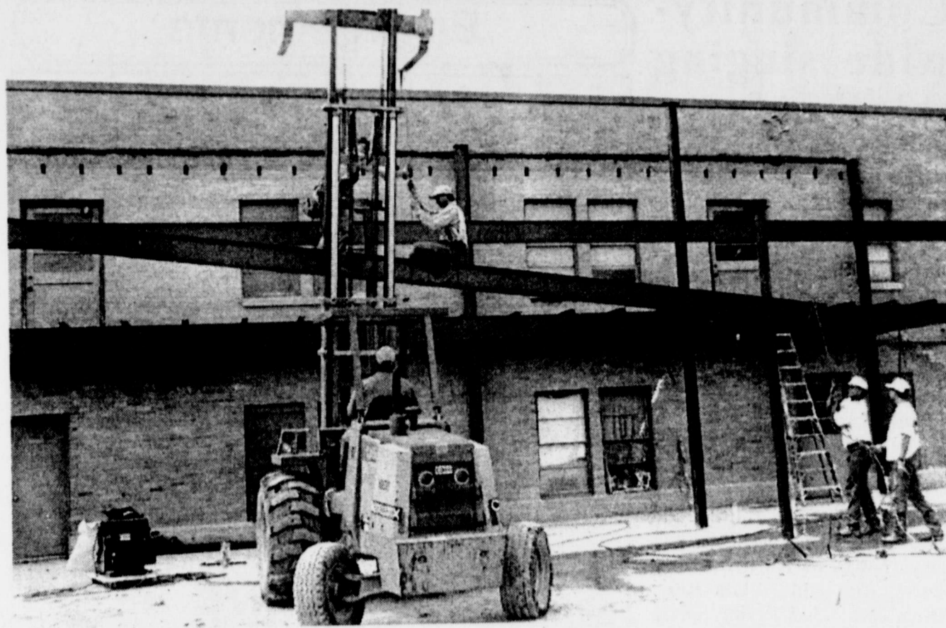
PROGRESS AT WINTERS FIRST BAPTIST CHURCH FELLOWSHIP HALL is beginning to be evident after several weeks of delay. The steel currently being put in place was not available for eight weeks, but an expected completion date of February 1995 is now anticipated. This will coincide with the church's 105 anniversary in March 1995 if no additional delays are encountered.
