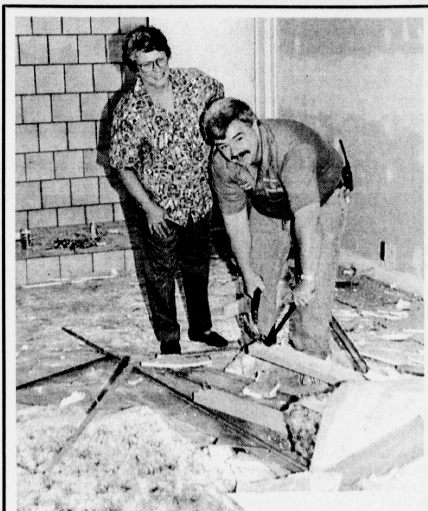
THIS IS HOW YOU USE A HAMMER...Jim Lincycumb and Georgia Jones survey the progress being made on the renovation of the old KRUN building on North Main where the new North
