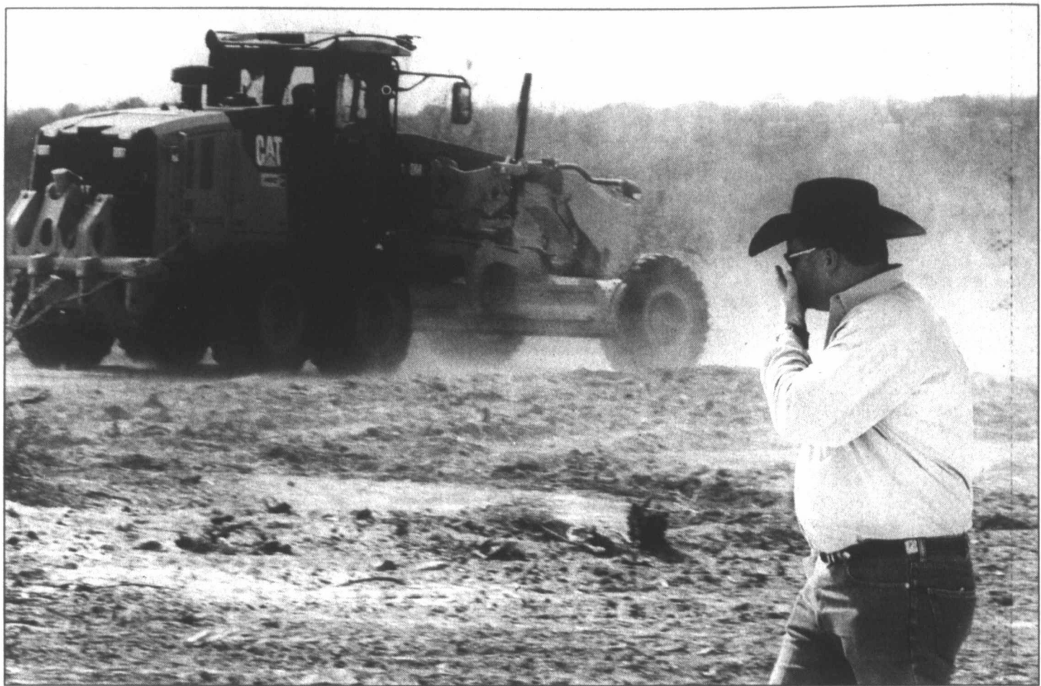
BREAKING GROUND — Todd Whitesides watches as one of Mine Services' employees works the land just south of I-20 and east of Hwy. 208. The land has been leased by Bridgeport Tank Trucks out of Bridgeport.
