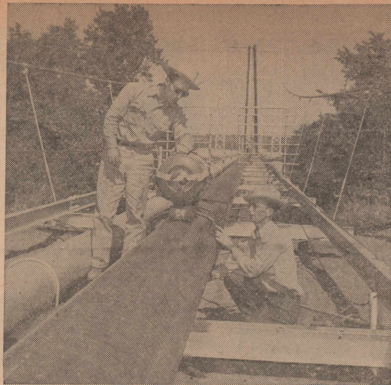
X-RAY UNIT was used to check welding on Lone Star Gas Company's new 20-inch line. Carrying 150,000 volts, unit provided film record which would show up any defects. Picture was made on Byers suspension bridge linking Texas and Oklahoma sections of new line. Expansion loops, background, were still incomplete.
