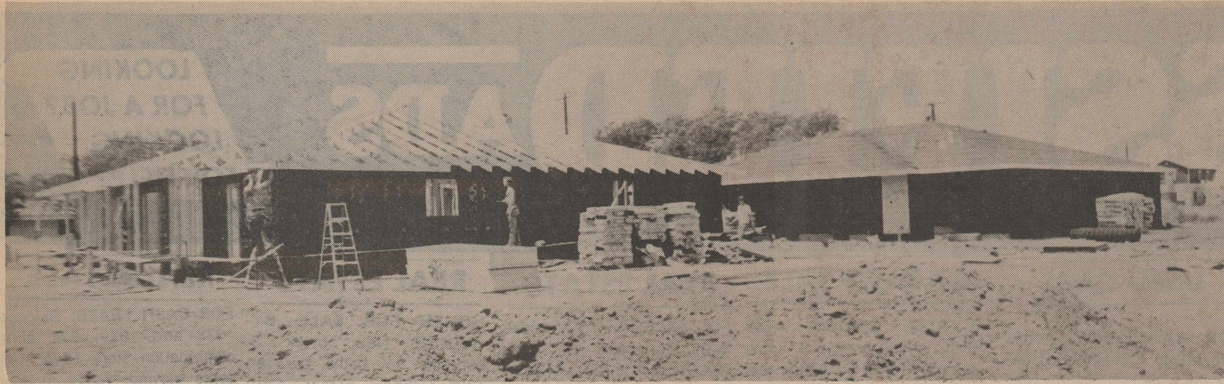
SAGEBRUSH II Construction is moving rapidly on these two four-unit apartments under construction on Corsicana Street between 8th and 9th. Owner and builder is Lev Connor of Dalhart, who is also the owner of Sagebrush I.
