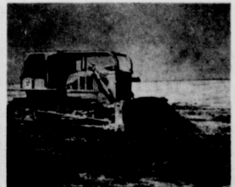
After removing the lignite, we begin to reclaim the land immediately. Within months it can be used to raise crops . . .
