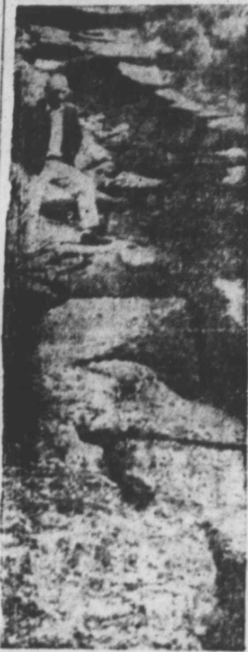
Center Line A forestry worker stands near a crack in the road at West Yellowstone, Mont., following the earthquake that struck the area.
