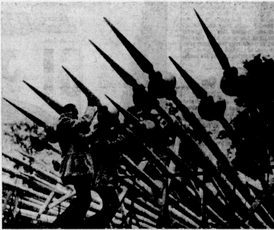
THEY'RE NOT WHAT THEY SEEM —Workmen prepare spearheaded gilded poles for erection around Buckingham Palace and in the Mall in London to honor the state visit to England by Portugal's President, Gen. Craveiro Lopes. The Portuguese leader is slated for a three-day stay.
