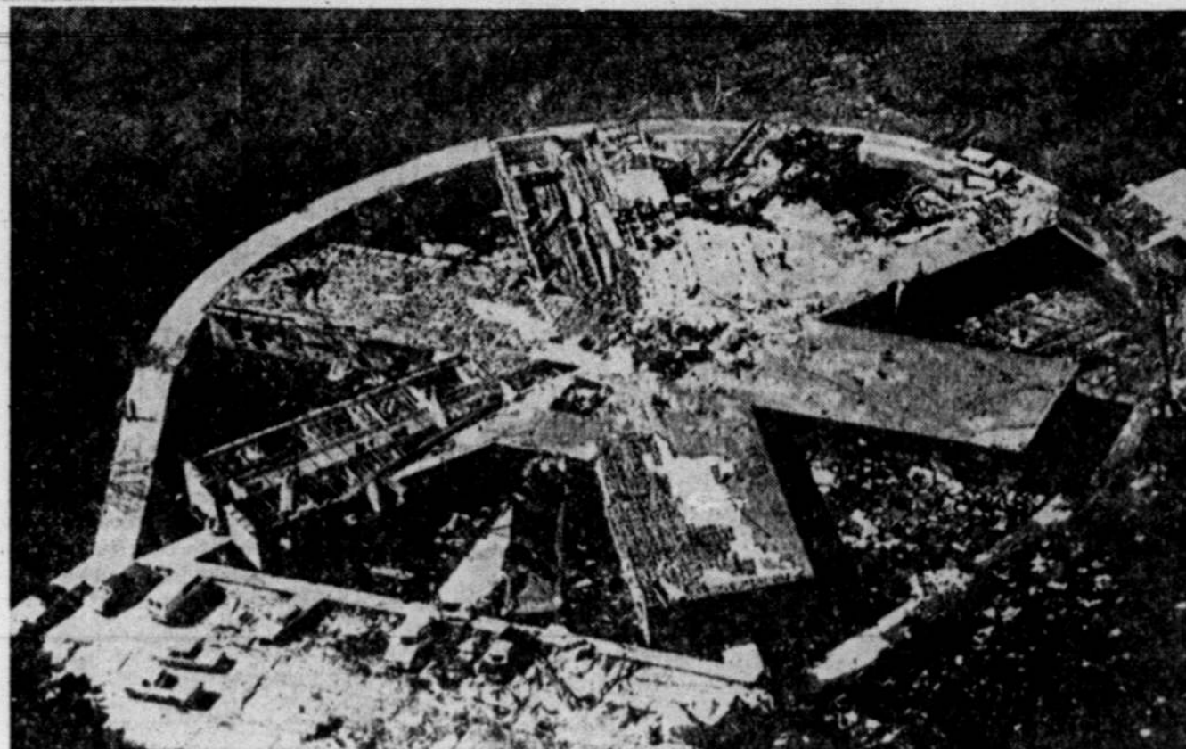
DIRECT HIT — Half the roof from Leisure Lodge Nursing Home in Hamburg, Ark., was ripped away by tornado that struck the commun-
