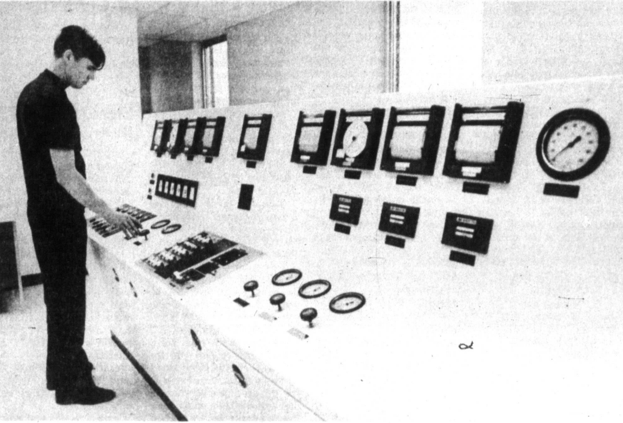
JUST THE PUSH OF A BUTTON —Tony Anderson, water superintendent of the Pampa Municipal Water Treatment Plant, pushed a button about 11:30 a.m. today to begin the flow of Lake Meredith Water into the city's distribution system. The lake water will be distributed on a
