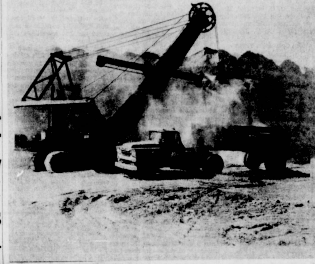
A MOUNTAIN OF CALICHE is being used in the reconstruction of Highway 62 from Floydada to the Crosby County line. This week-end scene indicates how a big shovel is used to load out an unending line of dumptrucks to take material to the road bed. Strain Bros. of San Angelo have the contract for the 10.8 miles of roadway at a price of $664,241.05. (Staff photo and engraving)
