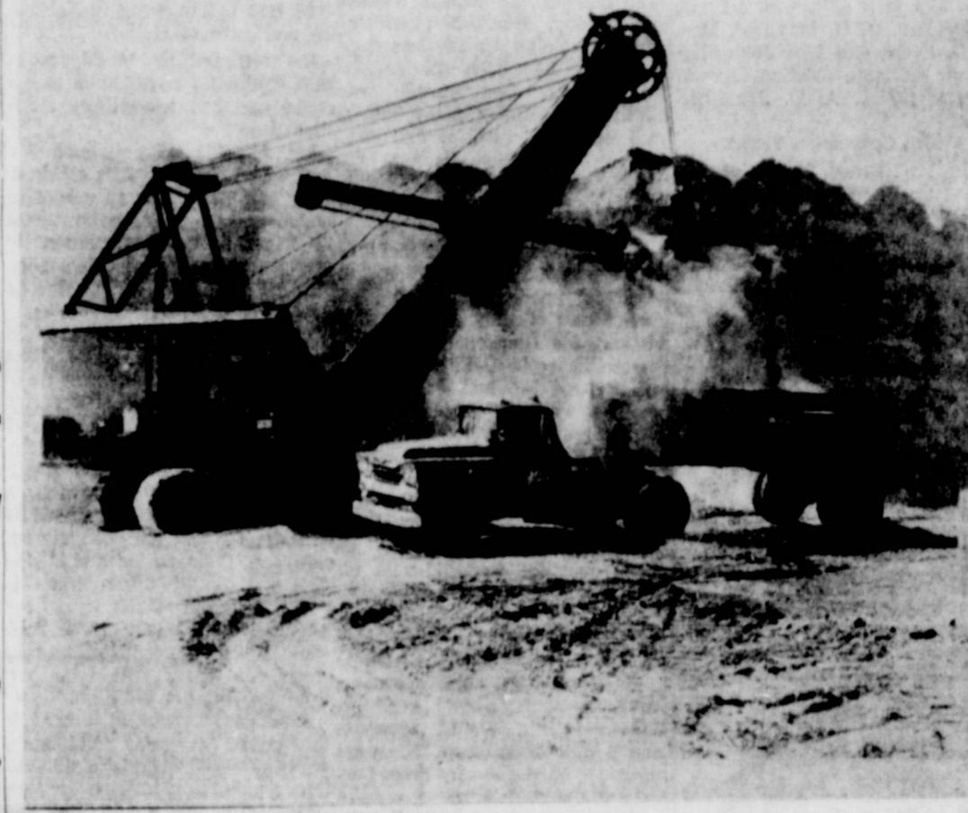
A MOUNTAIN OF CALICHE is being used in the reconstruction of Highway 62 from Floydada to the Crosby County line. This week-end scene indicates how a big shovel is used to load out an unending line of dumptrucks to take material to the road bed. Strain Bros. of San Angelo have the contract for the 10.8 miles of roadway at a price of $664,241.05. (Staff photo and engraving)
