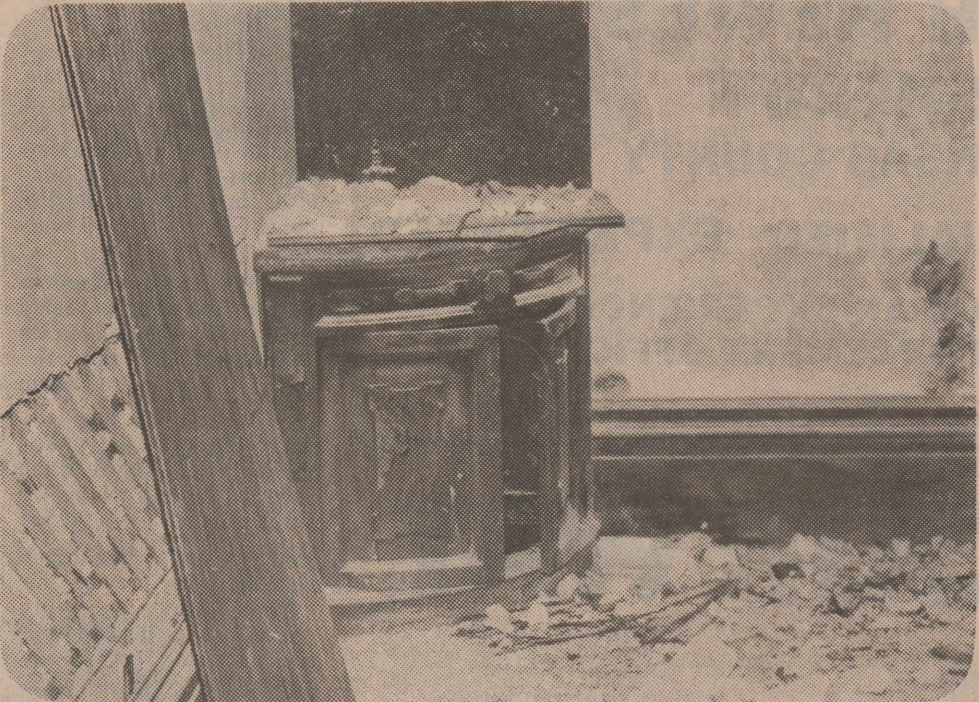
WORK NEEDED HERE
