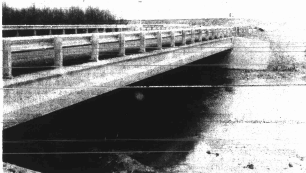
NEW BRIDGE IN SERVICE — Martin County traffic can now use the recently opened bridge on FM 846 at Sulphur Draw. The old structure was wiped out by flood waters on Sulphur Draw in June of 1987. Construction of the new bridge was delayed by continuing water problems. The Highway Department project was completed at a cost of $219,000.
