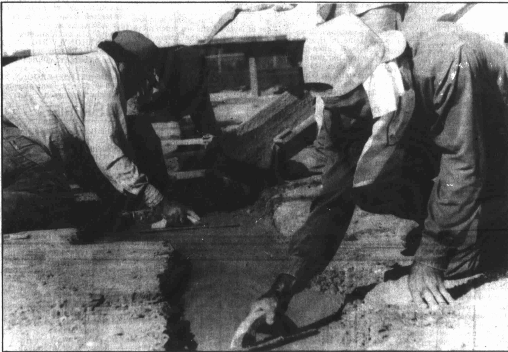
Gonzalo Billalobos, Frank Mendoza and Jose Granillo lay concrete at the new multi-purpose athletic facility at Big Spring High School. The three are employed by N.C. Sturgeon Inc. of Midland.
