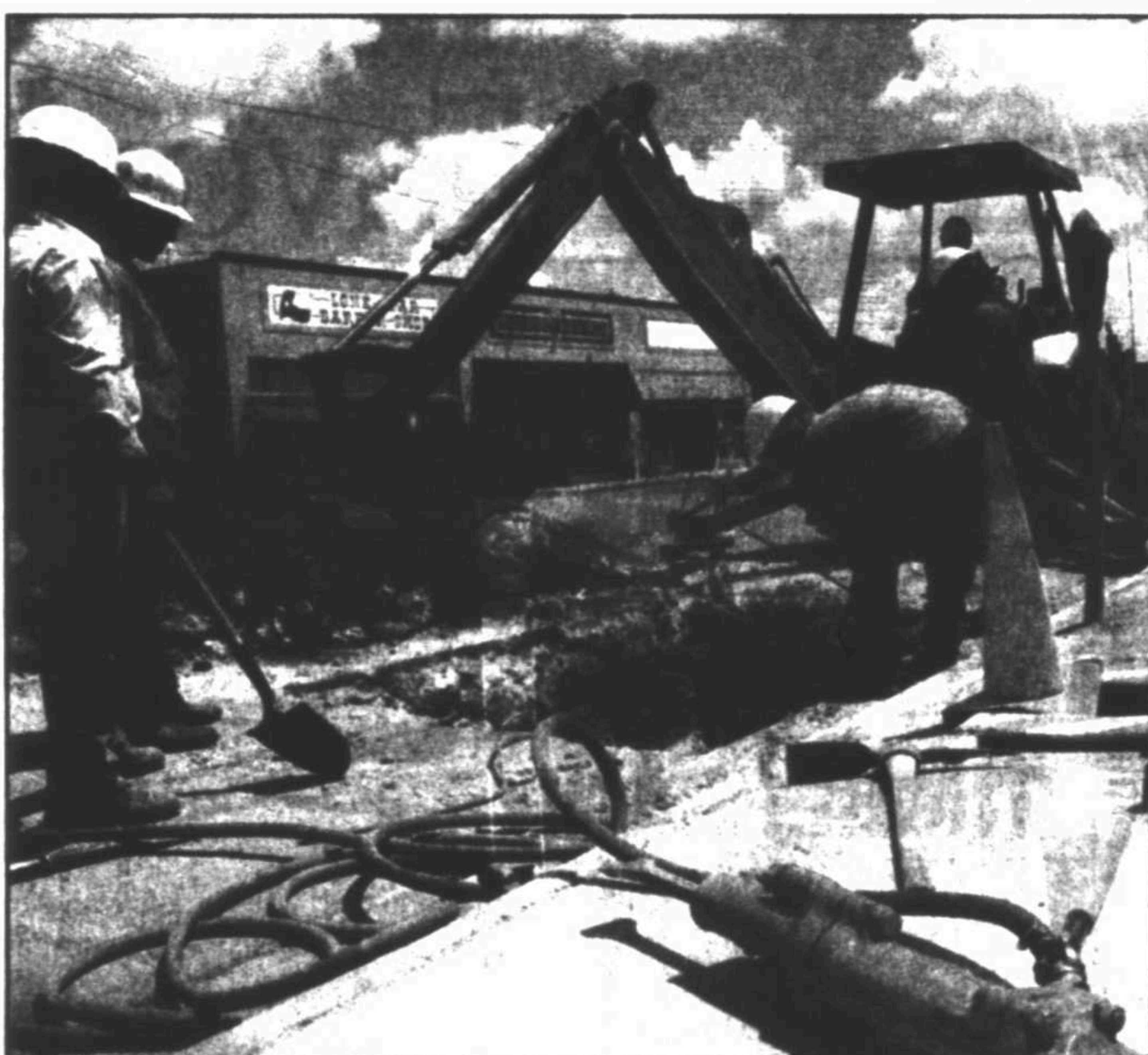
Crews gouged this massive hole on Wall Street to allow technicians access to a severed telephone cable. The cut cable left all of downtown without communications.
