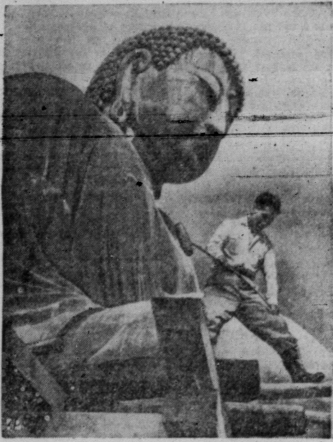
SHORING UP —The base of the Buddha at Kamakura, Japan, is reinforced to make it earthquake proof. The statue was elevated for a steel and concrete foundation.
