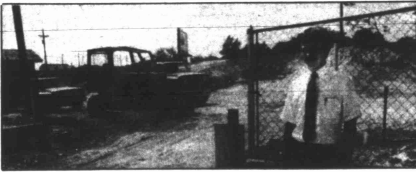
BIG SPRING — Ralph Johnson, the manager of the Golden Corral stands in front of a lot that is being leveled as part of an expansion project at the restaurant. The lot will become the parking lot, with the building being expanding into the current parking lot. No starting date on the building expansion has been named, but it could begin as soon as Thanksgiving.
