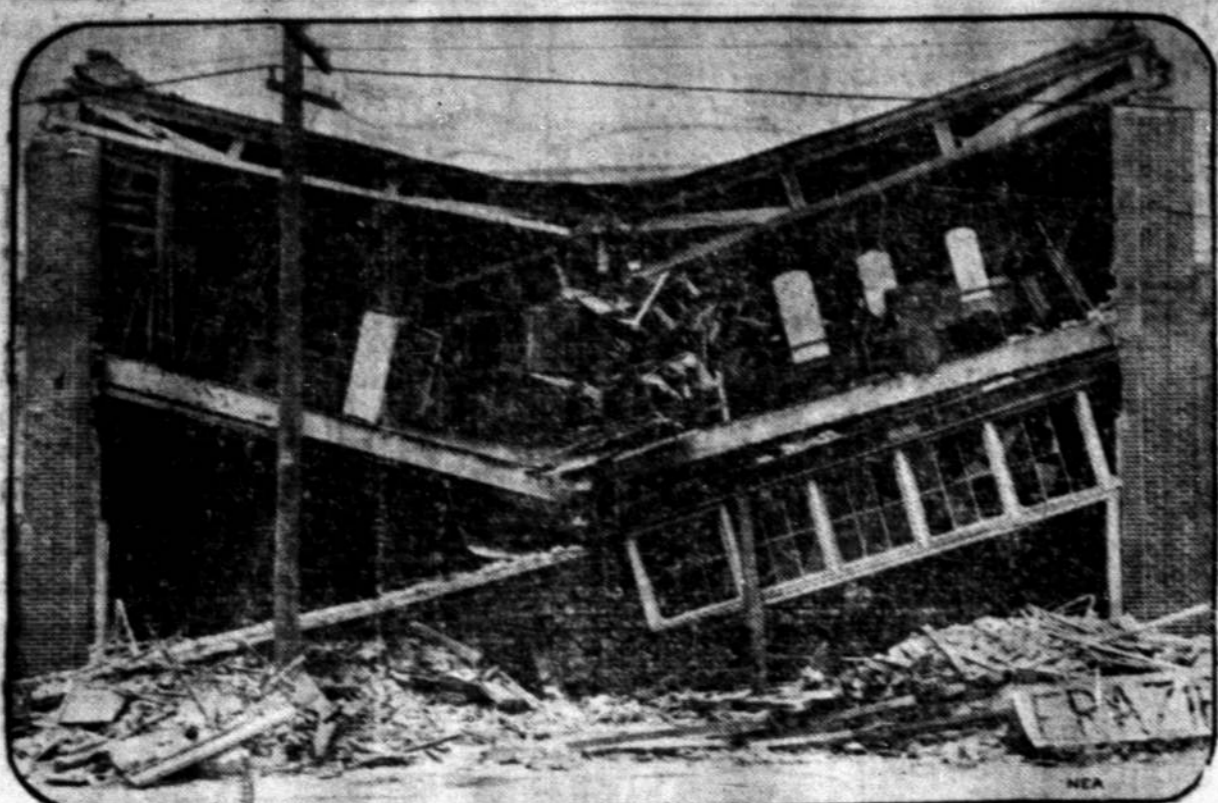
A one-man street car in Dallas, Tex., jumped the tracks and went on a rampage, crashing into the front of this furniture store and bringing so much wreckage down about it that it was two hours before it could be freed. The one-man crew, Everett Harrison, the car's only occupant, was unhurt.
