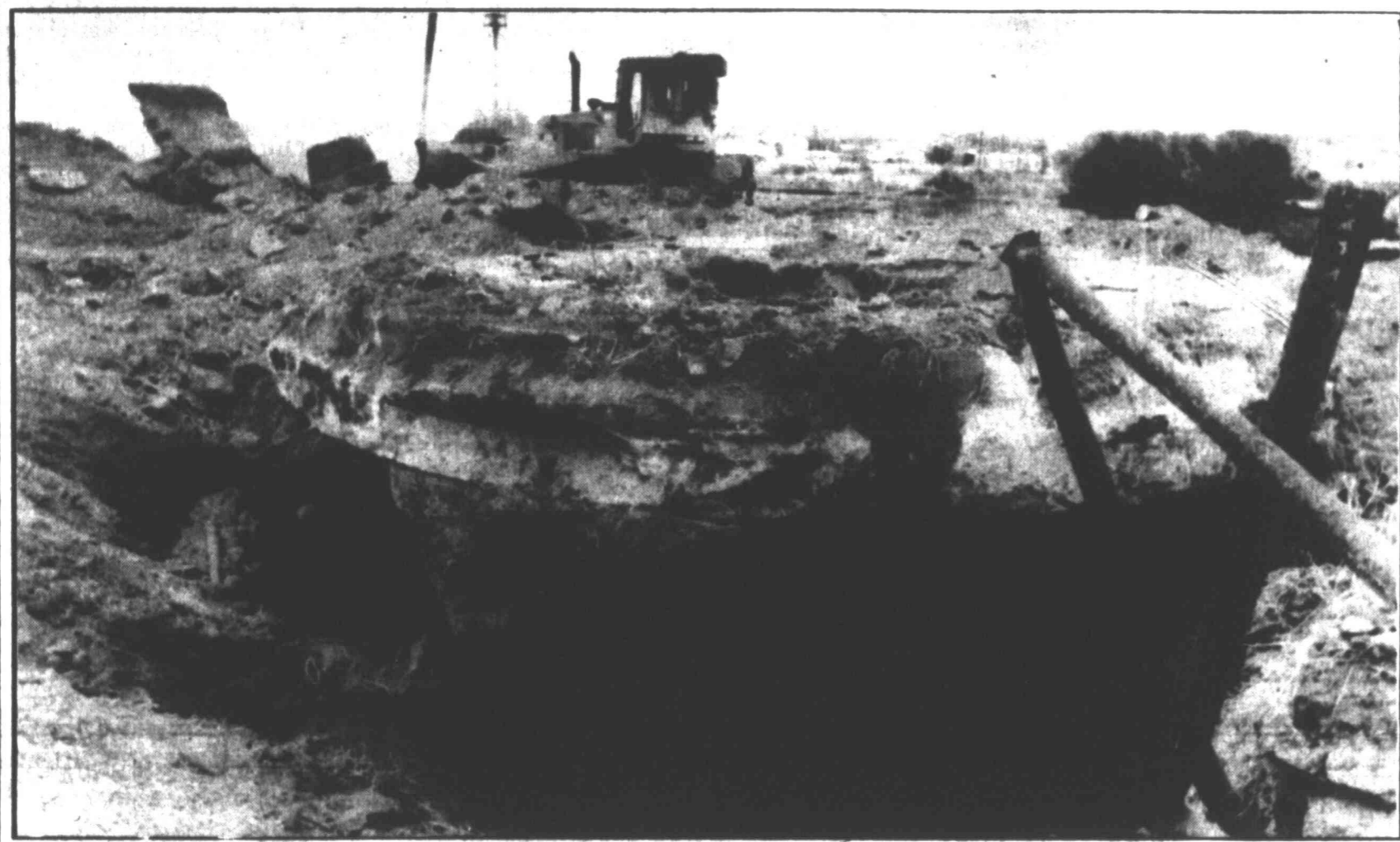
A bulldozer removes rubble from around the base of the old railroad water tower this week as the area near Beal's Creek is being cleared away as part of the creek widening project.
