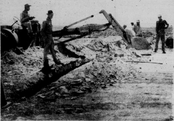
CUTTING THE CROSSING —New water and sewer lines are sprouting every block or so across Thirty-seventh Street as the deadline for completion of the project nears. When the job is completed, the State Highway Department will take over the street under their farm road program, widen and repave it.
