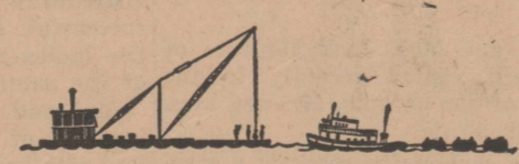
2,000-foot sections of pipe were shoved out into the lake, where tugs towed them to anchored barges.
