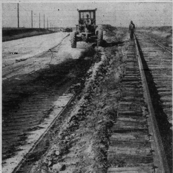
CONSTRUCTION CONTINUES on U. S. Highway 84 through Scurry County the cost of which will be over $5 million with county taxpayers paying only about $200,000 of the 4-lane project. Above, maintainers prepare the road bed for the R5&P tracks 5 miles southeast of Snyder which will be moved over to make room for the extra two lanes under construction alongside the existing pavement. Among other paving projects in the county are the widening and paving of Thirty-seventh Street and the "rodeo road."
