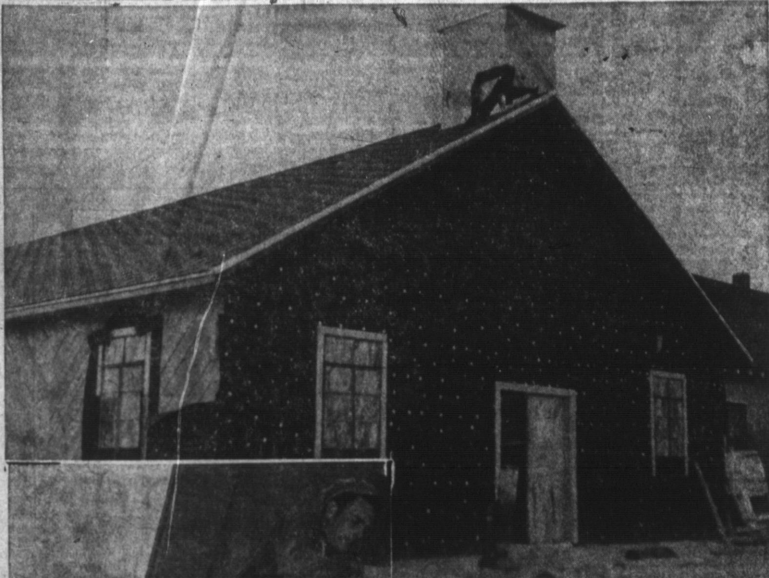
MEMBERS PITCHED IN to build the new, modern church nearing completion at Summerfield. The building, top photo, will be finished in brick veneer in around six weeks. LEFT PHOTO shows Guy Waiser and Reese Dawson in the foreground, two of a score of interested workmen.
