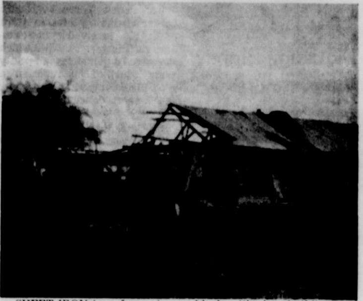
SHEET IRON torn from pioneer blacksmith shop building on Eubank Street, near city water tower.
