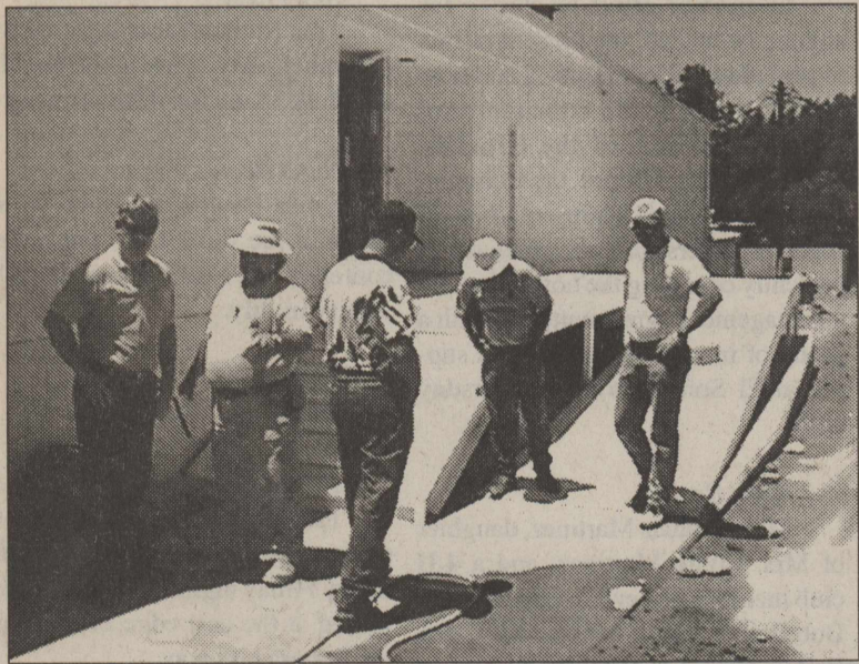
ARCHITECT LARRY HARVEY (far left) and engineer Jimmy May discuss the details of completing the handicapped access on the south side of Davidson Gymnasium. Principal Donnie Wylie, Maintenance Supervisor Ray Don Myers and Calen Easterwood survey the concrete work during the tour of the facilities. Photo by Scotty Moore.
