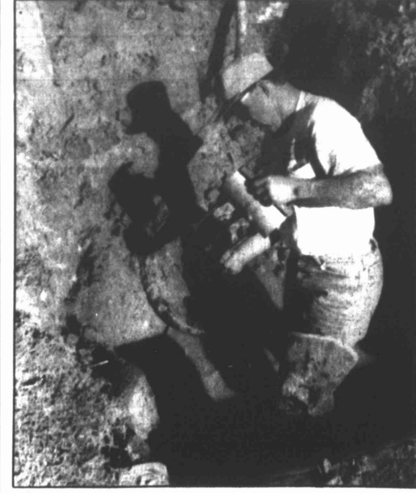
A City of Big Spring worker prepares to repair a broken water line along Scurry St. Thursday morning. Since the freezing weather last week, several water lines have needed repairs.
