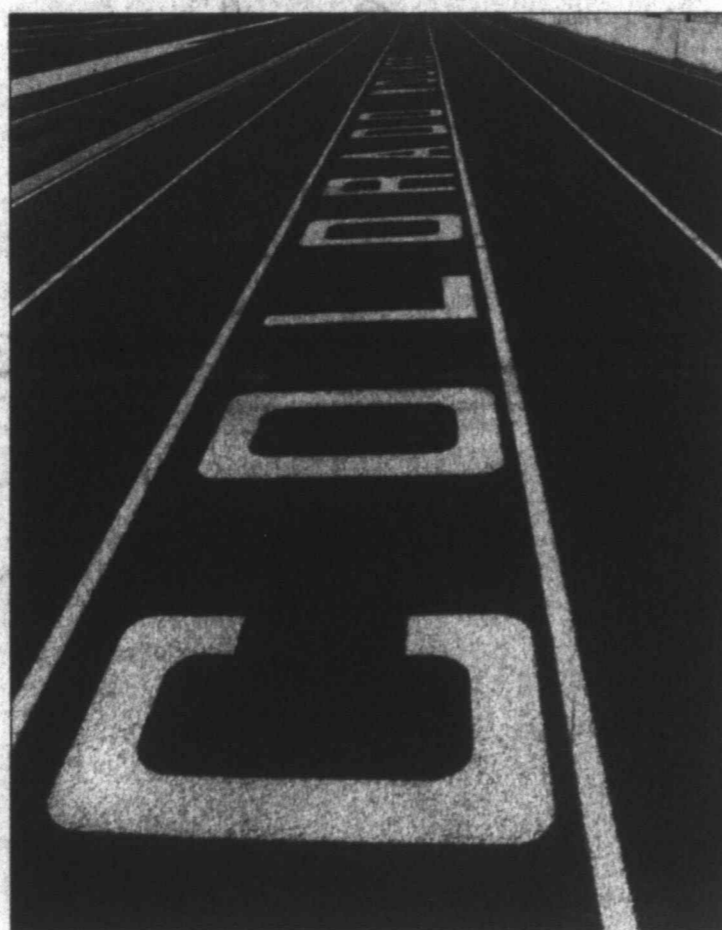
READY FOR TRACK - The Hollis Gainey Track at Wolf Stadium has been completely revamped and is finished in time for track season. The old running surface was dug up, a new surface put down and striping was completed last week.
