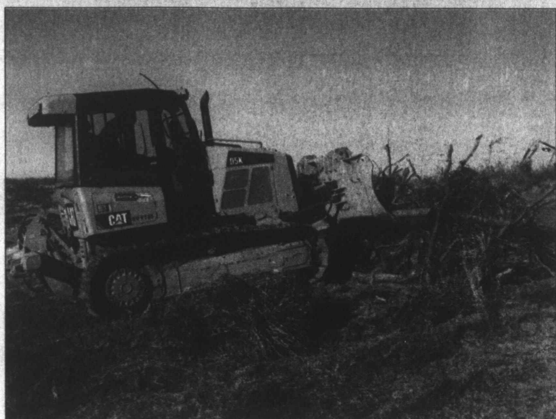
PLENTY OF SUN - Brush clearing has begun on 700 acres of land owned by Luminant on the northwestern side of Champion Creek Reservoir. Frankie Arguijo of Bolin Construction was hard at work clearing brush Monday, to make room for a planned solar farm. An attorney for the energy company has said he expects Mitchell County to be the location chosen for the project, if all continues to go well.
