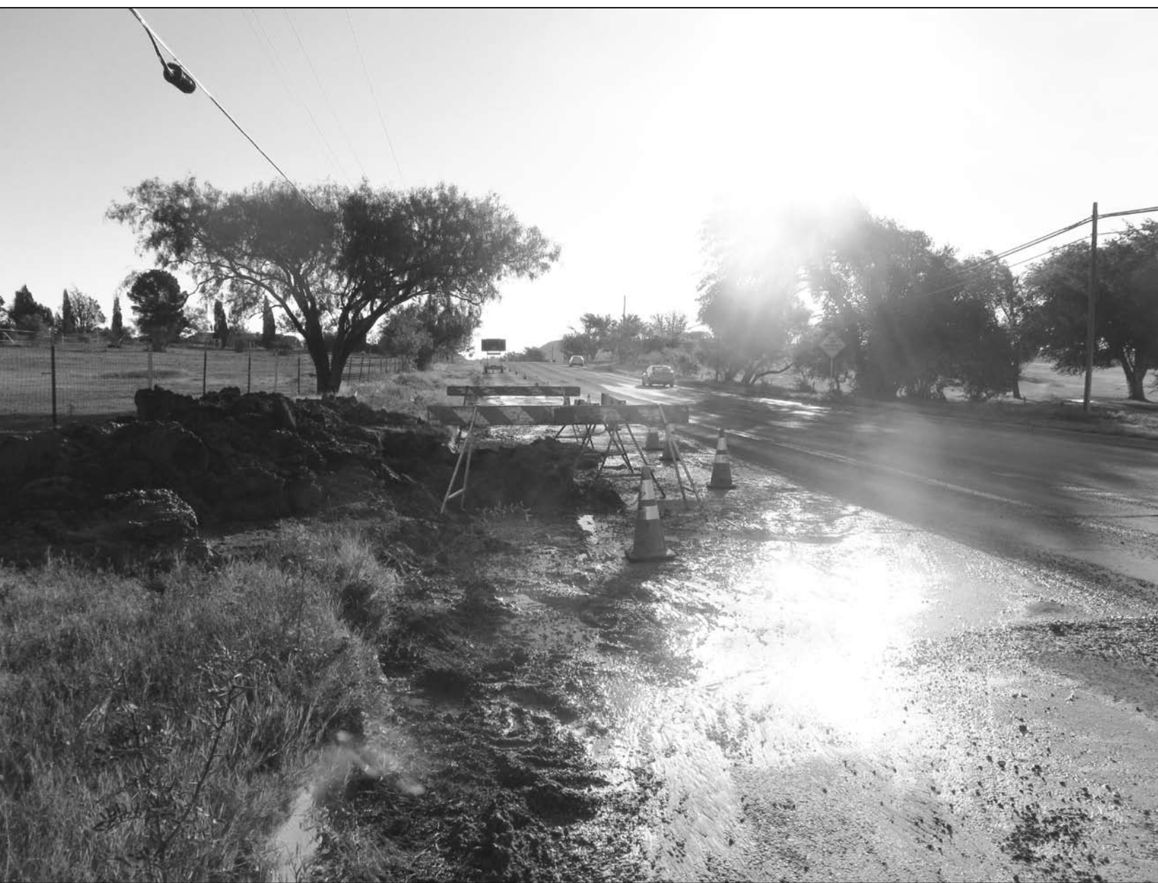
The city of Big Spring closed part of a lane on Wasson Road on Monday evening to tackle a water main break which occurred near Comanche Trail Park and Parkway.
