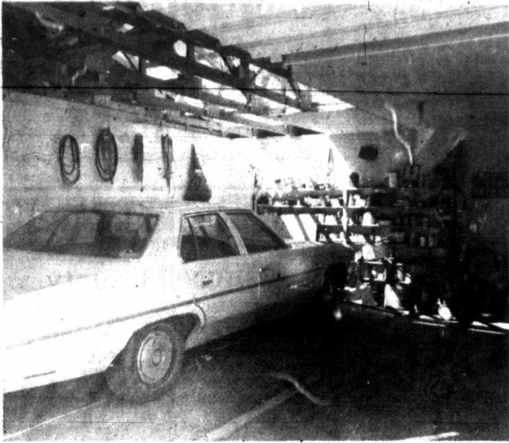
WEDNESDAY A TWISTER hit the Clarence Browne residence, causing extensive damage. Pictured is a portion of the garage roof which was torn off. Estimation of damages has not yet been made.
