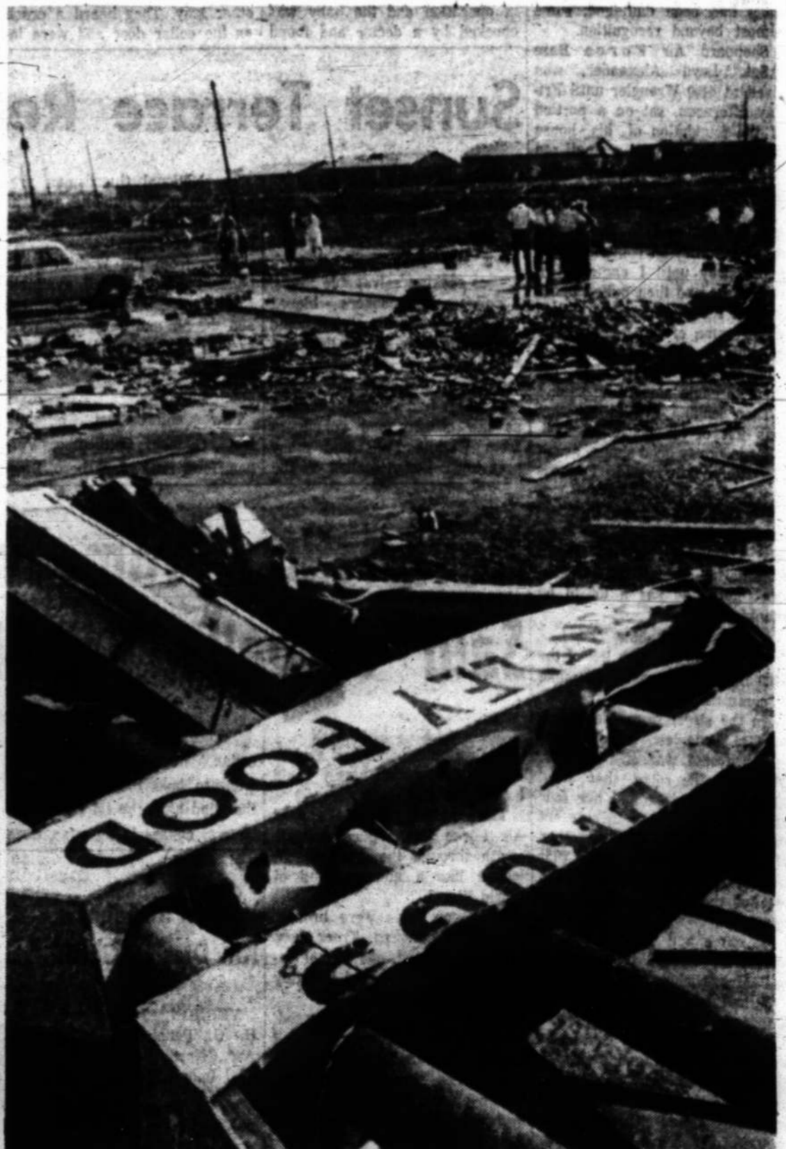
WAS FOOD STORE — The group of men in the upper center of the picture are standing on the concrete that was once a Seven-Eleven Food Store at 1722 Cimarron. The tower sign that stood on steel posts bedded in concrete is twisted in the foreground. Homes in the background are shown in various stages of damage from roof damage to leveled structures.
