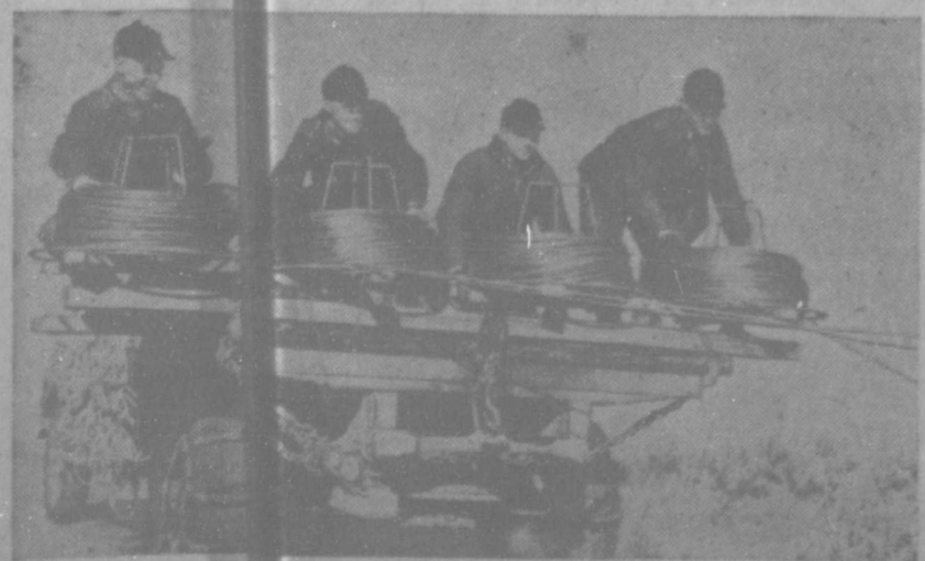
Stringing four lines of aluminum cable at once near Horton, Kan. REA projects have required 115,000 miles of this cable.
