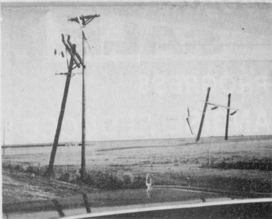
DARKNESS AFTER THE STORM -- While miraculously escaping a direct blow from the storm, Gruver was still without power at press time Friday because of storm damage such as
