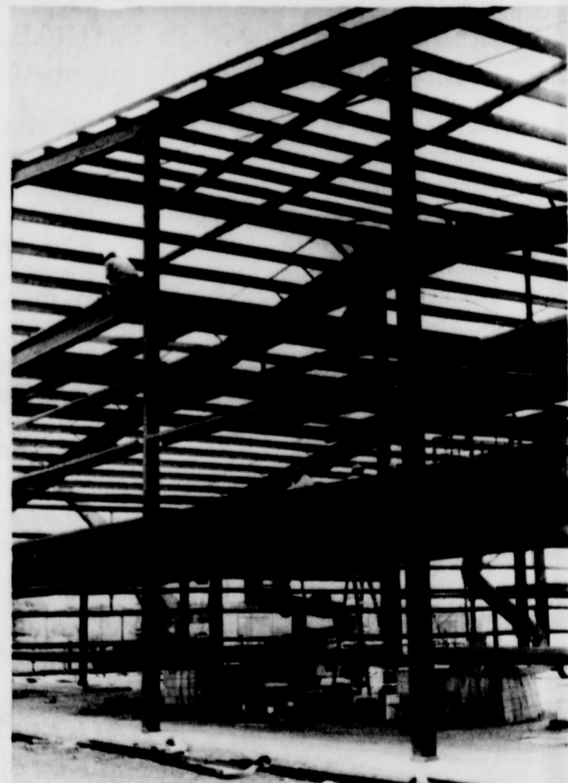
STEEL IS RAPIDLY GOING UP: Workers with Turner Construction are busy erecting the steel framing for the 334-bed dormitory-type facility within the walls of the 80-John Wallace Unit. About 30 employees are working on the building which will be completed in the summer.
