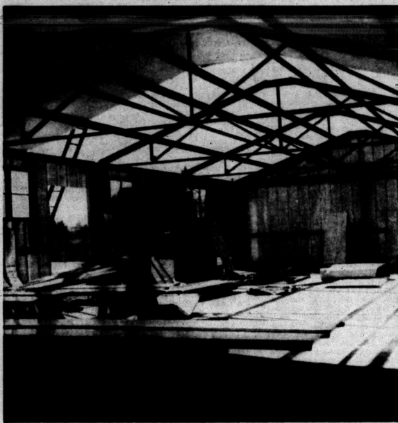
CONSTRUCTION WORK IS PROGRESSING on the new city shops and warehouse buildings being built on Thirty-seventh Street east of Avenue M. The building shown will be used for a repair shop, storage of water department supplies and storage of the emergency hospital equipment of the Civil Defense agency. The buildings will replace the old barn in the 1900 block of Twenty-seventh Street which will be removed to make room for the new fire, police, and civil defense operating center.
