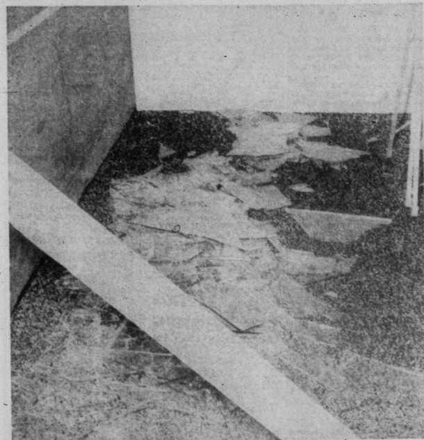
STORM DAMAGE —This window at J. C. Penney Co. and two more were victims of last night's wind. The other two were at Furr's Super Market and the Buccaneer Stamp Store.
