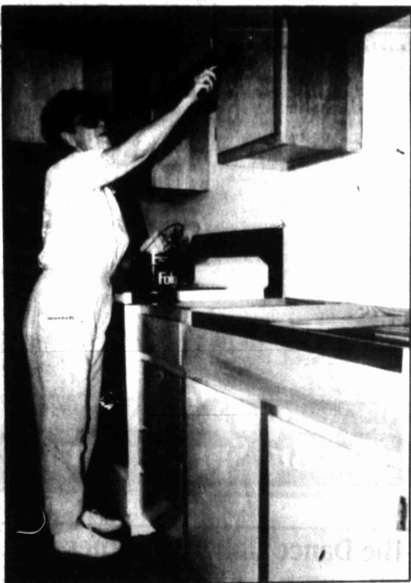
Babs Moore puts the finishing touches on the communal kitchen cabinets. Kitchen and dining room facilities provide space for cooking and eating should families choose to dine in. Emergency staples are on hand for families who can't afford their own food.
