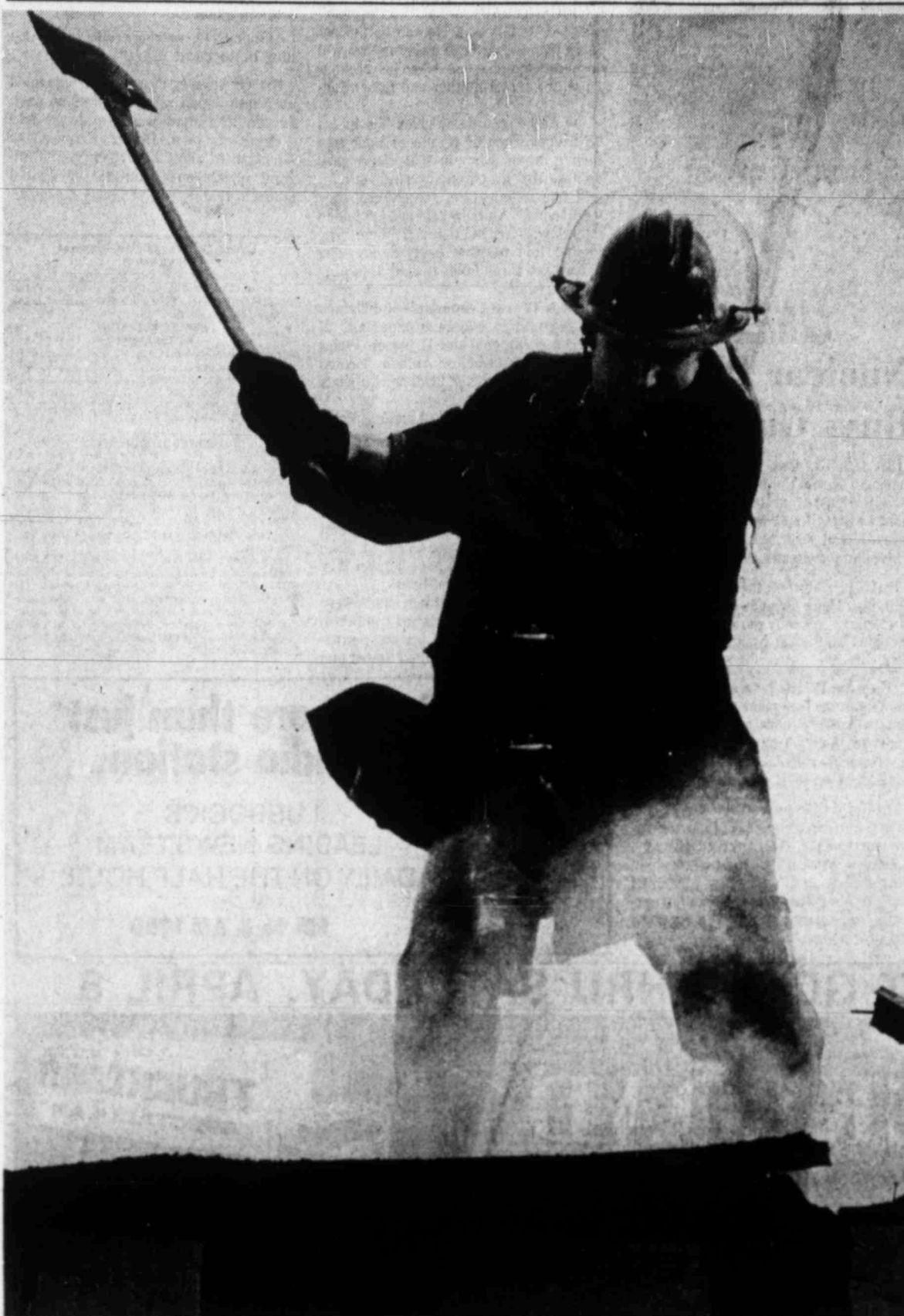
CUT IT DOWN! — Fireman Jim Shuey of Station 4 cuts through a smoldering roof at the Village Inn on the Brownfield Highway early this morning. No one was hurt in the blaze, but police ushered about 75 persons from the motel rooms. Investigators suspect the fire started in a pile of stored carpets behind the building's south wing. (Staff Photo by Paul Moseley)
