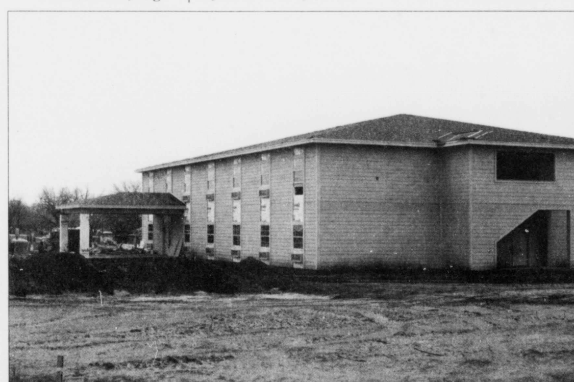
MOVING TOWARD THE final phases of construction, the new Westbrook Suites motel draws closer to a spring opening.
