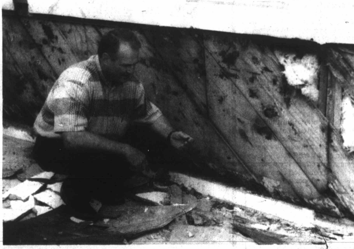
MITCHELL COUNTY HOSPITAL Maintenance Supervisor Sam Parham inspects the condition of the outside wall on the north wing. Maintenance crews were making repairs this week to stop water leaks that occur inside the building when there's even a small amount of rain. Insulation in the right corner of the exposed wall in this picture will be tested for hazardous materials this week by an outside survey team.
